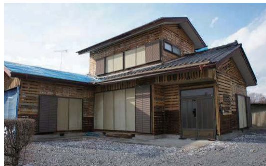
Photo 6.2-62 Damage of exterior mortar wall
