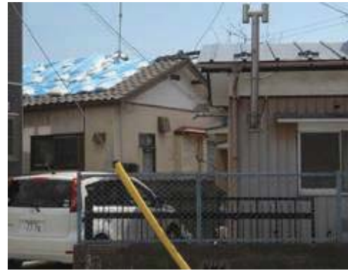
Photo 6.2-34 Damaged roof tile in Hiyorigaoka
