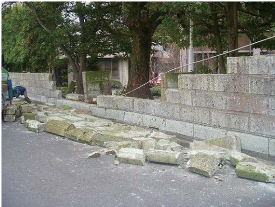
Photo 6.3-52 Collapse of stone masonry wall (Fukushima city)
