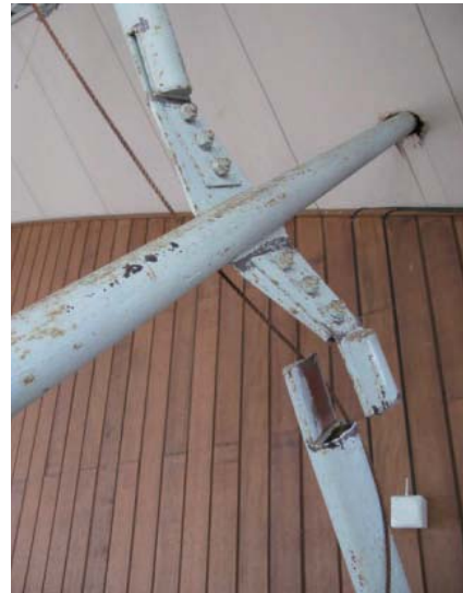
(b) Fracture at brace crossing
