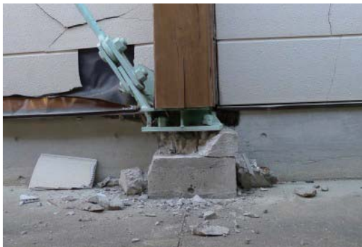
Photo 6.2-78 Breakage of the foundation concrete
