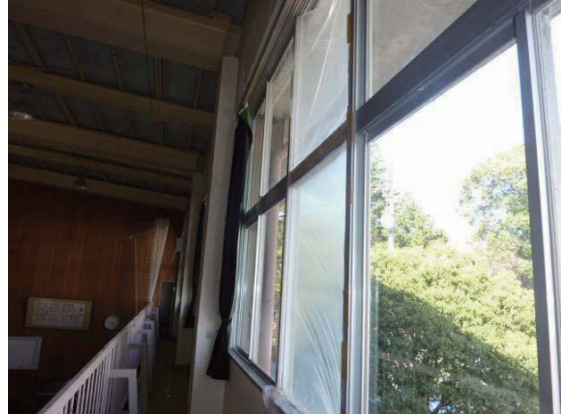
Photo 6.6-10 Breakage of window glasses installed to fixed window frame with glazing bead
