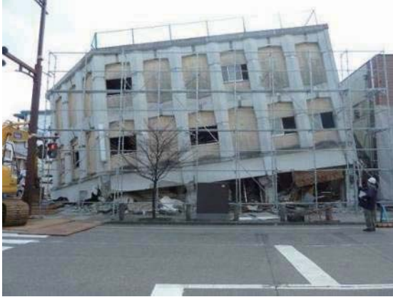
Photo 6.3-4 First-story collapsed building (Sukagawa city)
