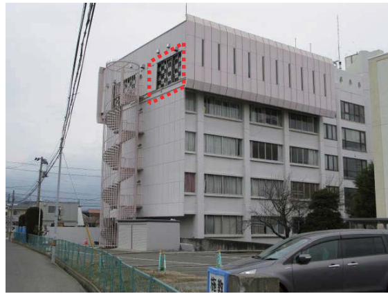
Photo 6.6-7 Detachment of AAC panels
