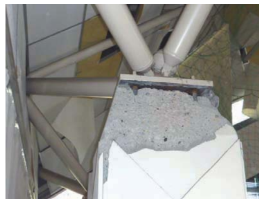
Photo 6.4-7 Spalling of concrete
