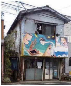
Photo 6.2-41 House with large residual deformation (Komatsujima)
