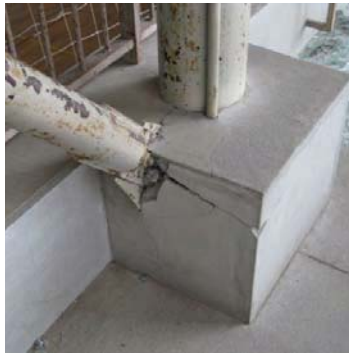
Photo 6.4-11 Cracking of column base concrete
