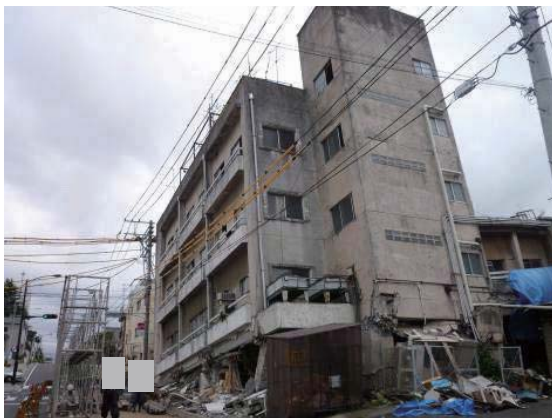
Photo 6.3-2 First-story collapsed building (Koriyama city)
