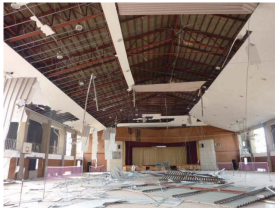
Photo 6.4-18 Dropping of extensive ceiling components
