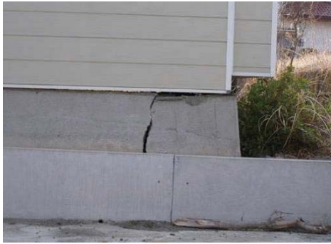
Photo 6.2-67 Crack of foundation
