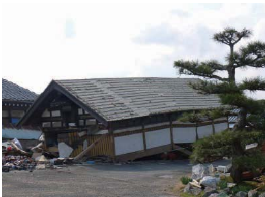
Photo 6.2-72 Collapsed nagayamon gate (Kadobe)
