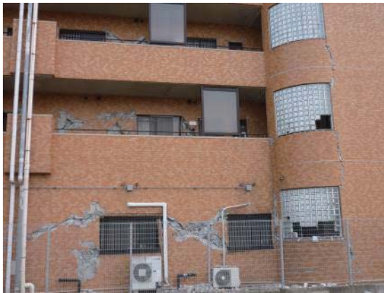
Photo 6.3-43 Damage of nonstructural wall in same building shown in Photo 6.3-22 (Koriyama city, Fukushima pref.)
