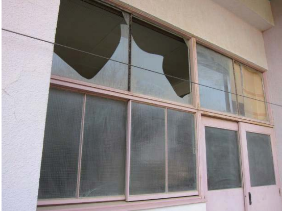
Photo 6.6-9 Breakage of window glasses installed to fixed window frame with hardening putty
