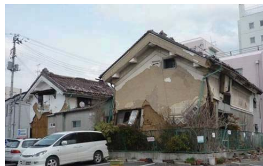
Photo 6.2-47 Failed warehouse with mud wall
