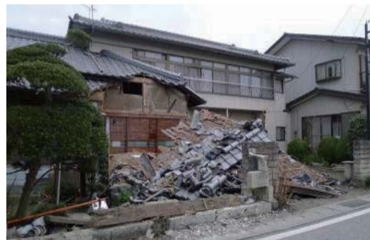
Photo 6.2-70 Breakage of entrance part.
