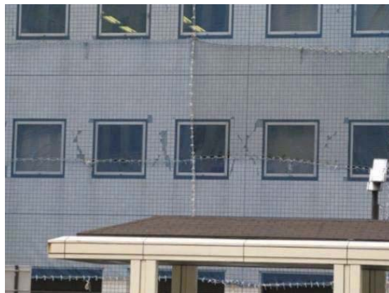
Photo 6.3-49 Damage of tile on exterior wall
