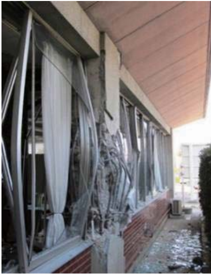
Photo 6.3-15 Shear failure of short column
