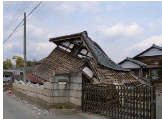
Photo 6.2-82 Damaged barn (Aoyagi-cho)
