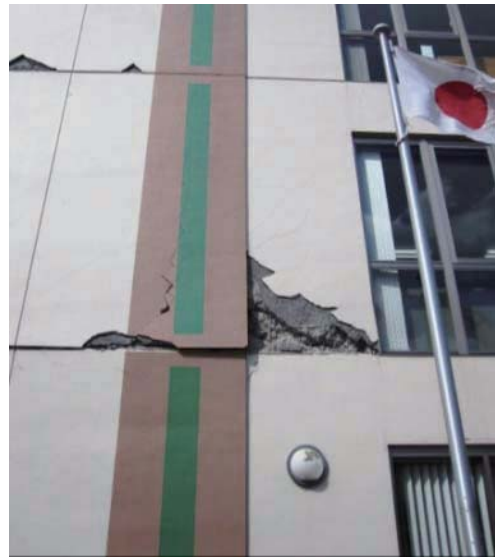
Photo 6.3-40 Separation of concrete of wing wall
