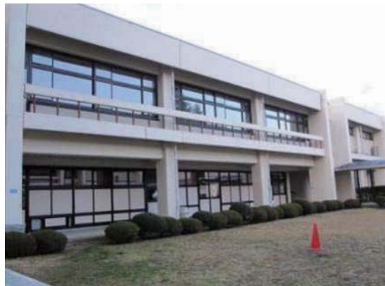
Photo 6.3-12 Appearance of the damaged building (Aoba ward, Sendai city)
