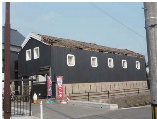
Photo 6.2-12 Warehouse with mud walls whose roof system with roof tiles fell down
