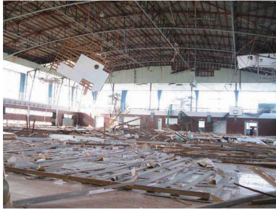
Photo 6.6-14 Falling of wooden suspended ceiling
