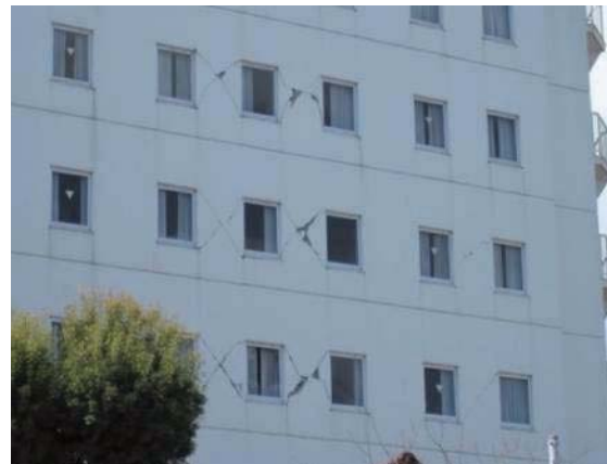
Photo 6.3-46 Shear crack on nonstructural wall
