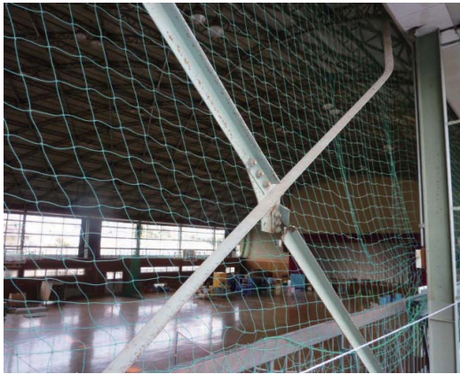
Photo 6.4-1 Buckling of brace
