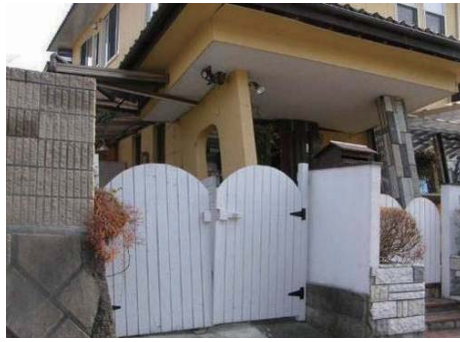
Photo 6.2-68 Wood house with large shear deformation
