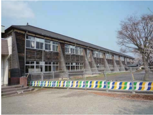
Photo 6.2-19 Seemingly slightly damaged School building
