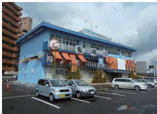
Photo 6.3-6 Mid-story collapsed building (Wakabayashi ward, Sendai city)
