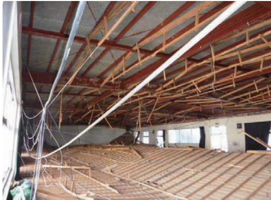
Photo 6.4-17 Dropping of extensive ceiling components
