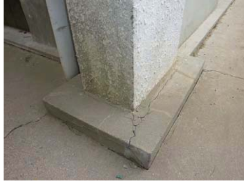
Photo 6.4-12 Cracking of column base concrete
