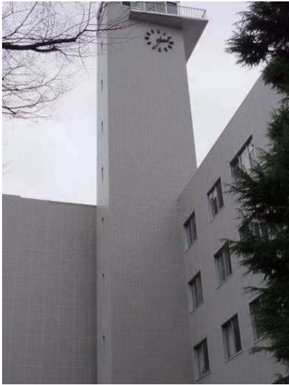
Photo 6.3-35 Damaged clock tower (Fukushima city)
