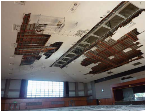
Photo 6.6-15 Falling of metal furring suspended ceiling
