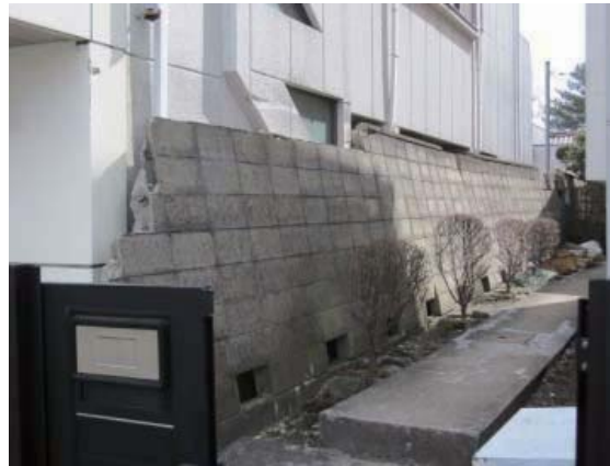
Photo 6.3-51 Collapse of concrete block wall (Sukagawa city)
