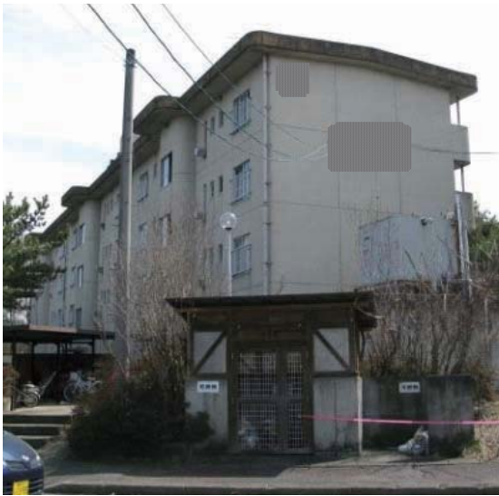
Photo 6.3-32 Appearance of sunken and leaned building (Shirakawa city)
