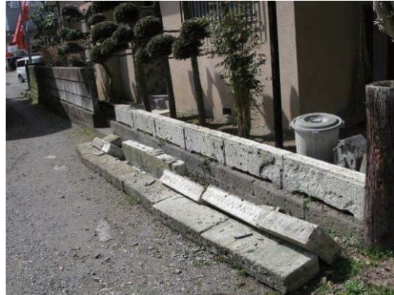
Photo 6.3-53 Collapse of stone masonry wall (Shirakawa city)
