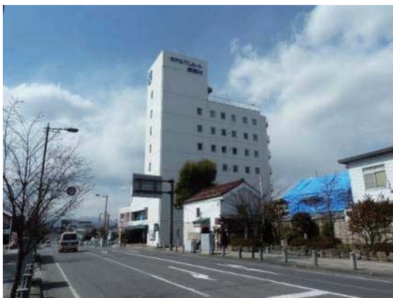
Photo 6.3-45 Appearance of damaged building (Sukagawa city)
