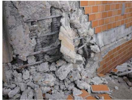
Photo 6.3-23 Damage at the bottom of SRC column
