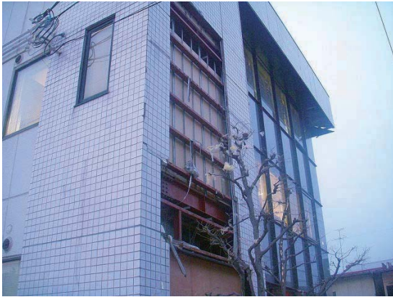
Photo 6.6-3 Falling of cement mortar and metal lath wall
