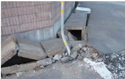
Photo 6.5-6 Damage to side ditch
