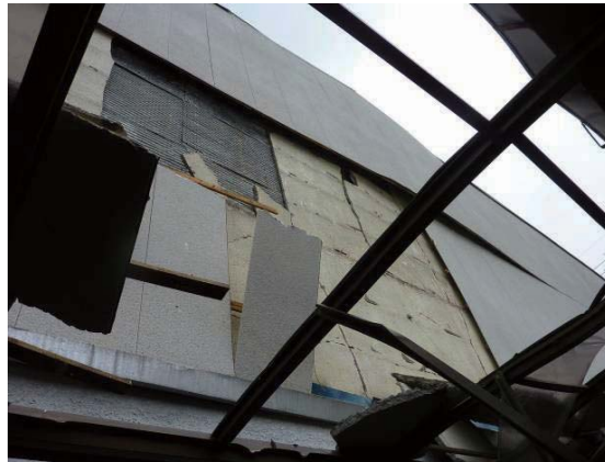
Photo 6.6-5 Damage to gymnasium gable end wall
