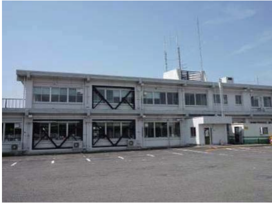
Photo 6.3-37 Appearance of damaged building (Hitachiomiya city)
