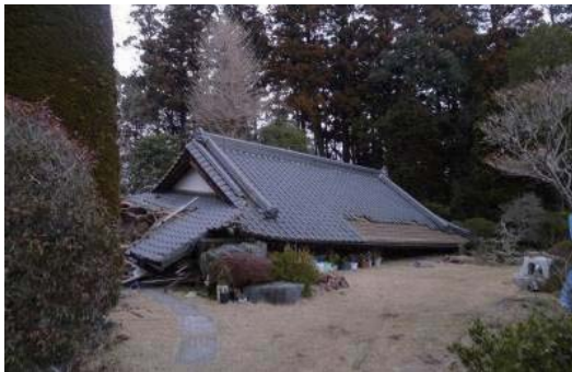
Photo 6.2-69 Collapsed wood house
