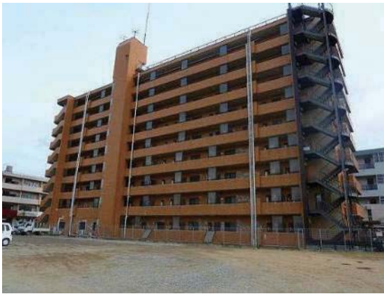
Photo 6.3-22 Appearance of damaged building (Koriyama city)
