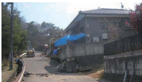
Photo 6.5-13 Damage to retaining wall and house due to sliding and ground deformation
