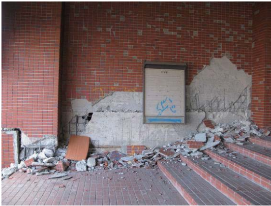
Photo 6.3-25 Damage of the bottom of SRC column and shear wall
