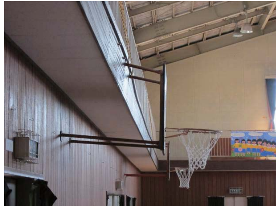
Photo 6.6-25 Damaged interior wall
