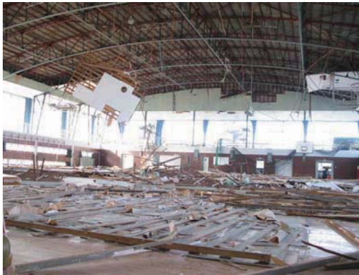
Photo 6.4-16 Dropping of extensive ceiling components
