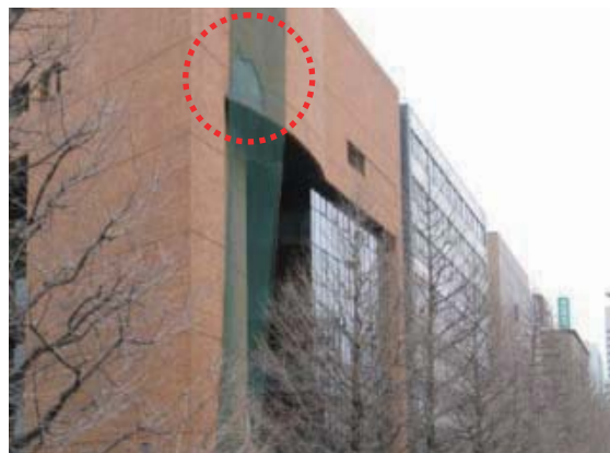
Photo 6.6-2 Detachment of ceramic wall tiles from RC wall
