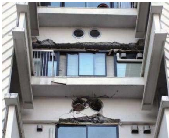
Photo 6.3-28 Damage of boundary beam with opening
