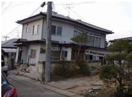
Photo 6.2-39 Damage of house caused by the ground transformation (Oritate)
