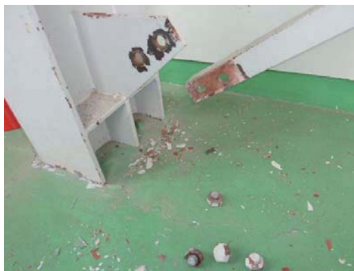
Photo 6.4-4 Fracture of bolts
