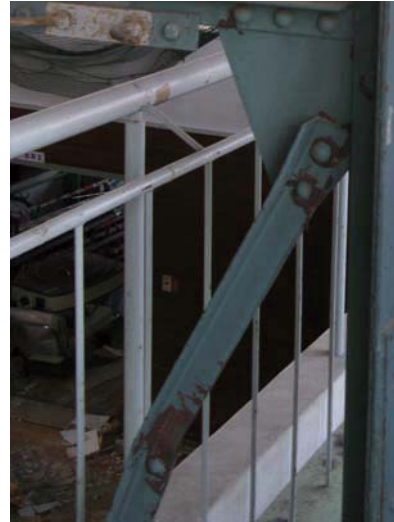
(b) Buckling of diagonal member
