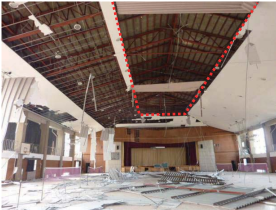
Photo 6.6-17 Falling of metal furring suspended ceiling and corrugated steel plates
