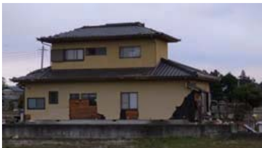
Photo 6.2-71 Falling down of mortar plastered wall
