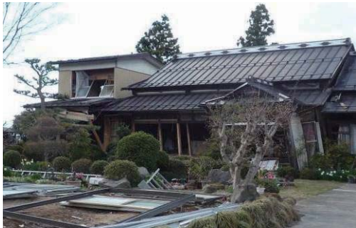
Photo 6.2-23 Largely tilted house
