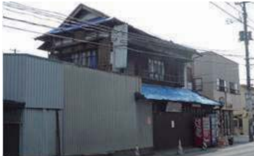
Photo 6.2-21 House with store with 2 nd story drift more than that of 1 st story
