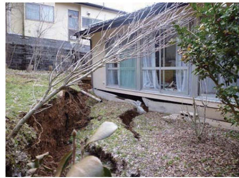
Photo 6.2-38 Damage of house in Photo 6.2-37
