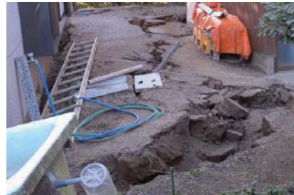
Photo 6.5-5 Crack in the site
