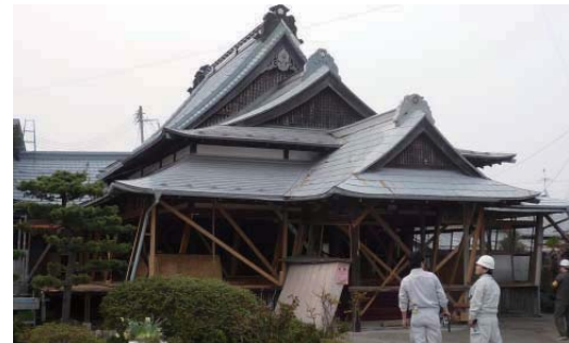
Photo 6.2-22 Heavily damaged temple building
