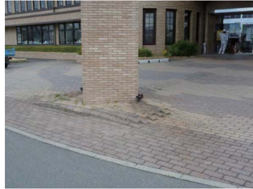
Photo 6.2-30 Ground deformation in Nango branch town office
