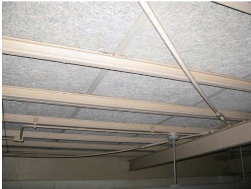
Photo 6.4-9 Deflection of horizontal braces
