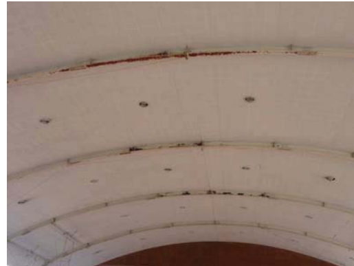
Photo 6.4-14 Peeling of paint of beams
