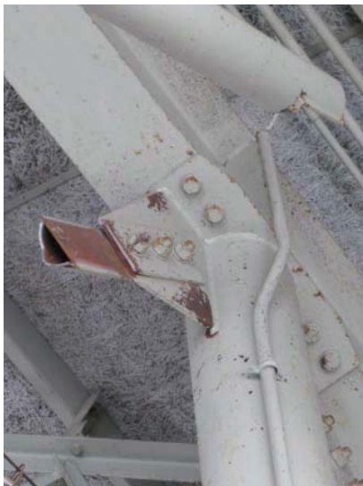
(a) Fracture at column top
