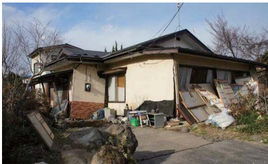
Photo 6.2-63 Wood house with large story drift
