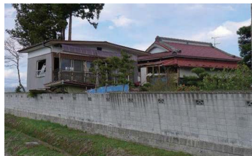
Photo 6.2-24 Collapsed wood house
