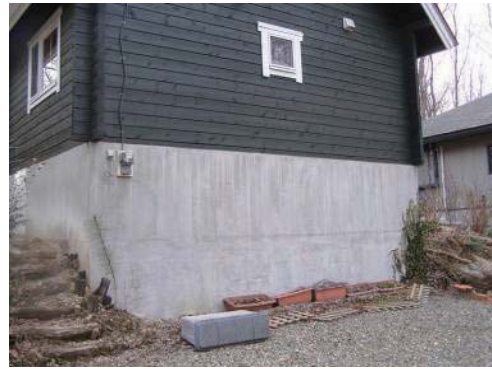
Photo 6.2-60 Crack of foundation
