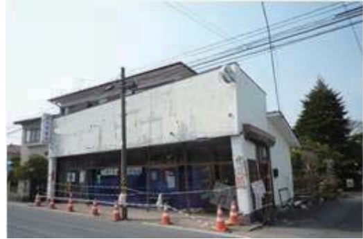
Photo 6.2-20 House with store with large story deformation
