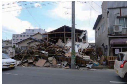
Photo 6.2-35 Collapsed wood house
