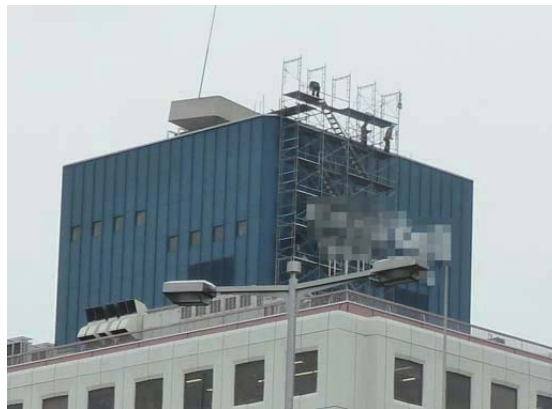
Photo 6.3-34 Damaged penthouse (Aoba ward, Sendai city)
