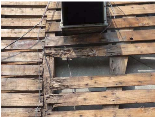
Photo 6.2-15 Deterioration in building of Photo 6.2-14
