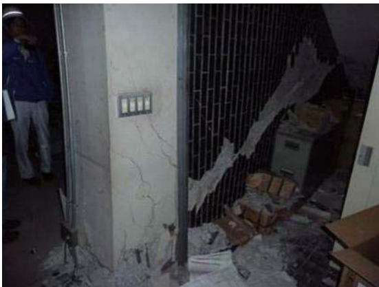
Photo 6.3-10 Shear crack on shear wall
