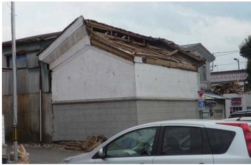
Photo 6.2-48 Fallen roof of warehouse with mud wall
