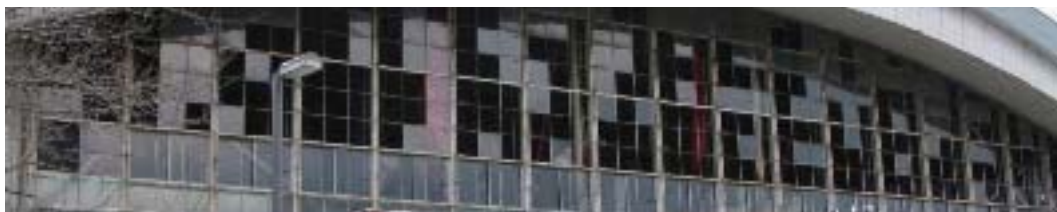
Photo 6.4-19 Breakage of windows
