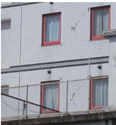
Photo 6.6-1 Detachment of ceramic wall tiles from damaged RC exterior wall
