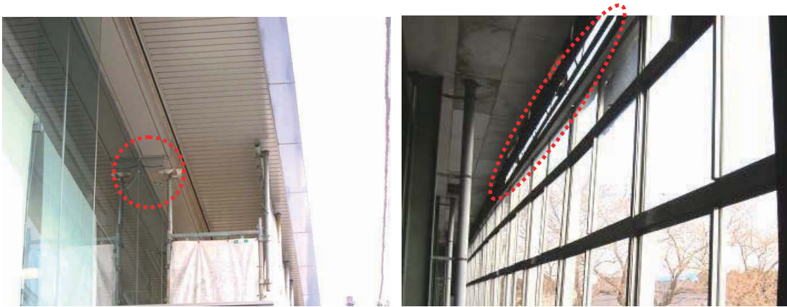
Photo 6.6-12 Breakage of glass mullion of glass wall system Photo 6.6-13 Dislocation of window frame
