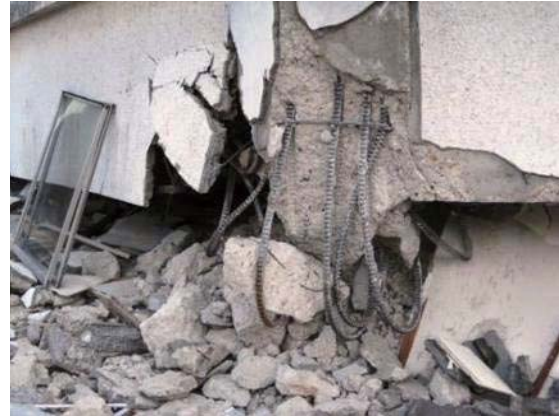
Photo 6.3-5 Close-up view of the fallen story
