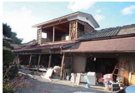
Photo 6.2-28 Largely tilted wood house
