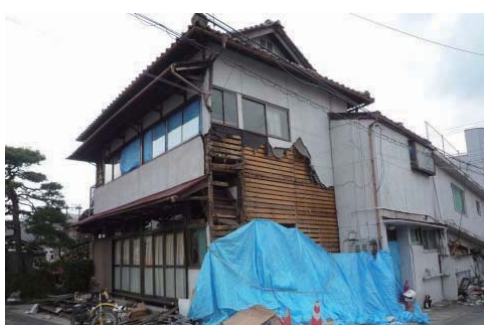
Photo 6.2-46 Collapsed stair hall
