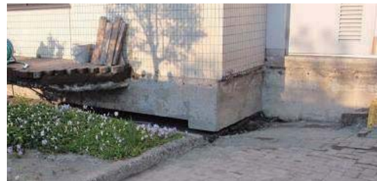
Photo 6.5-12 Building with subsidence of surrounding ground
