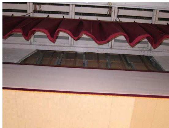
Photo 6.6-23 Falling of cement mortar finish above stage
