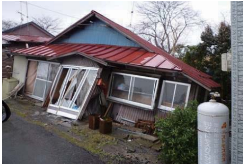
Photo 6.2-3 Damage of houses caused by ground transformation
