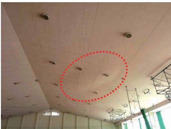
Photo 6.6-19 Sagging of metal furring suspended ceiling
