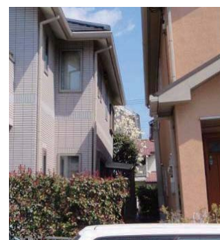
Photo 6.5-10 Settled and tilted house
