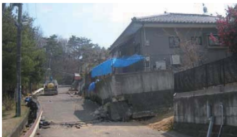
Photo 6.5-13 Damage to retaining wall and house due to sliding and ground deformation
