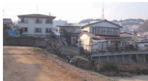
Photo 6.5-14 Group of houses damaged due to sliding and ground deformation
