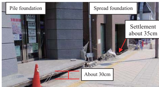
Photo 6.5-11 Difference in damage due to support mechanisms
