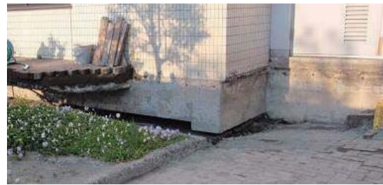
Photo 6.5-12 Building with subsidence of surrounding ground
