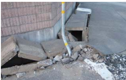
Photo 6.5-6 Damage to side ditch
