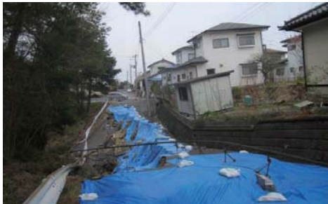
Photo 6.5-17 Fracture of embankment retaining wall and houses tilting due to land sliding on the slope of hill end
