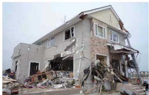
Photo 7.4-19. Light frame construction wood house (12) remained alone
