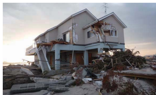
Photo 7.4-23. Mixed structure which has 1 st story of RC structure and wooden 2 nd story.
