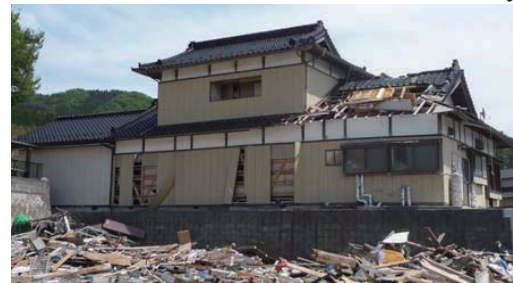
Photo 7.4-30. Wood house (6) which was not carried away in spite of damage on 1 st floor roof system in Akasaki-cho, Oofunato city.
