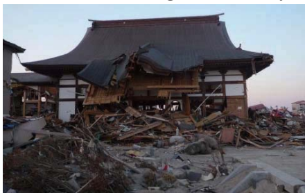
Photo 7.4-12. Heavily damaged temple ( 3 ) building in Yuriage, Natori city.
