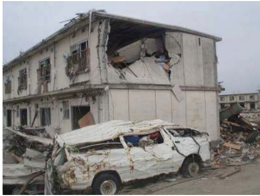
Photo 7.2-6 Wall opening probably generated by debris impact
