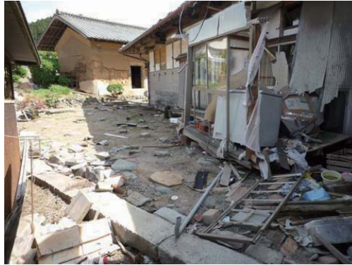
Photo 7.4-33. Survived old house (12) which rotated and moved horizontally in Akasaki-cho, Oofunato city.
