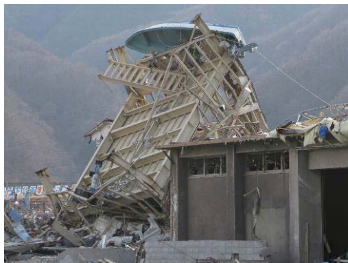
Photo 7.2-7 Steel building overturned by fracture of column base anchor bolts
