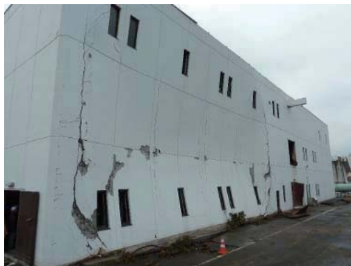
Photo 7.2-5 Out-of-plane fracture of reinforced concrete shear wall without floor
