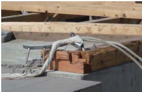
Photo.7.4-5. Failed hold down fastener.
