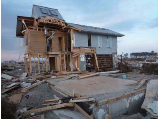
Photo 7.4-24. L-shaped wood house whose part was washed away in the east of Arahama port.
