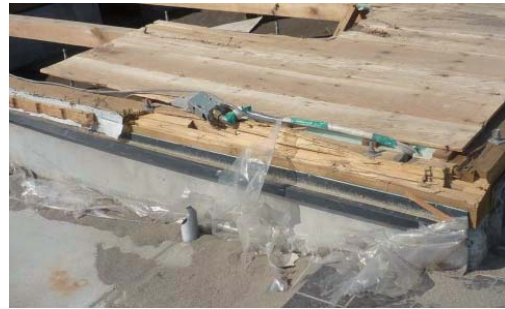
Photo.7.4-4. Sills, foundation and floor boards remained.
