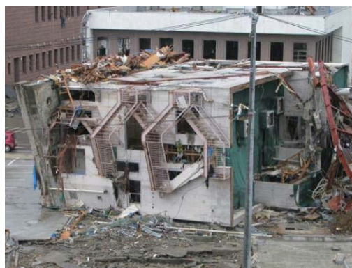
Photo 7.2-9 Overturning of a 3-story steel building
