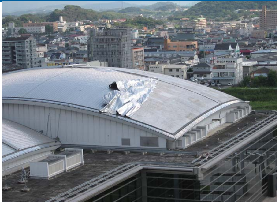
Photo 3. The roof of the Iizuka Cosmoscommon in Fukuoka Prefecture damaged by Typhoon Shanshan in September 2006
