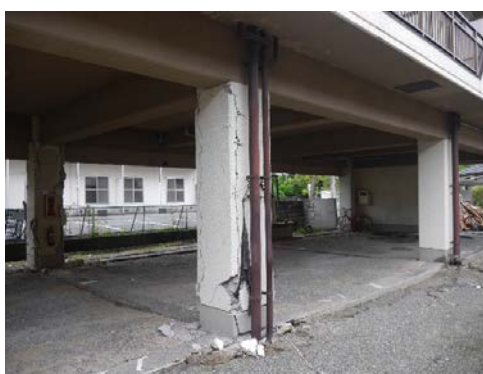
写真5.5-14 X3-Y1 柱 (付着割裂破壊、損傷度IV)
