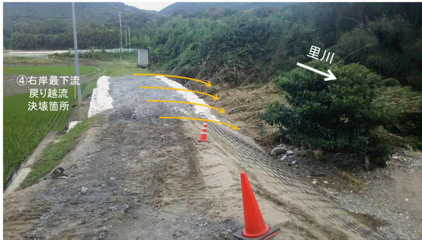
写真-5.2.6.16 ④右岸最下流決壊箇所の状況
