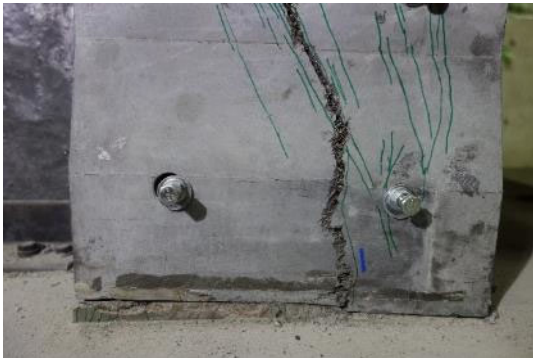
(c) 柱下目地モルタル圧壊
