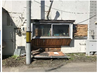
(c) 壁の崩落
